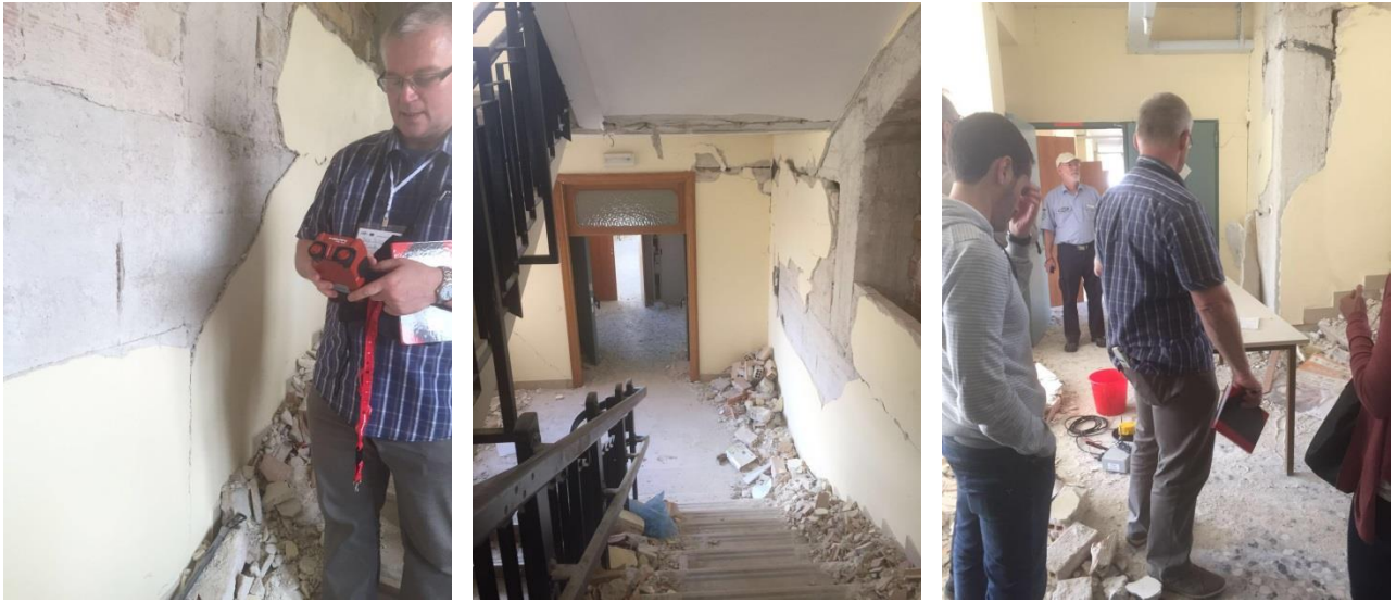
Figure 2: Some images of the building surveyed as part of the demonstration of the methods under development within SIBYL.
